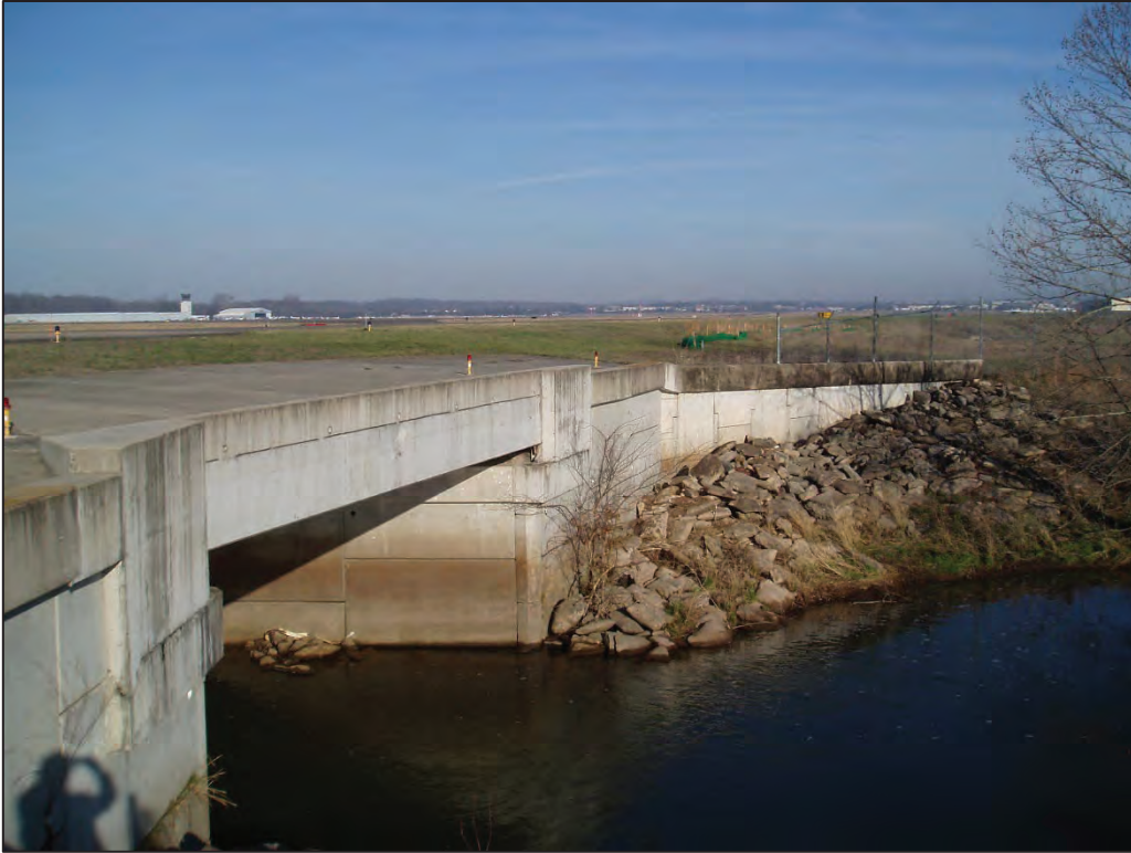
Photograph 17. The existing east side of the Cannon Branch bridge structure underlying T/W B (Field Photograph CSW_P3140005, 03/14/2024).
