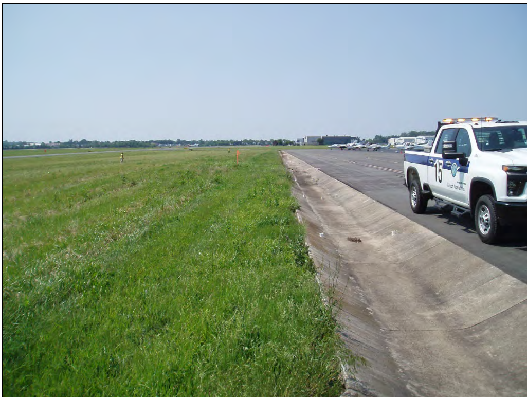
Photograph 8. Looking N at the west edge of the East Ramp and its existing drain. The bioswale as depicted on the concept includes part of the grassed area to the west.
