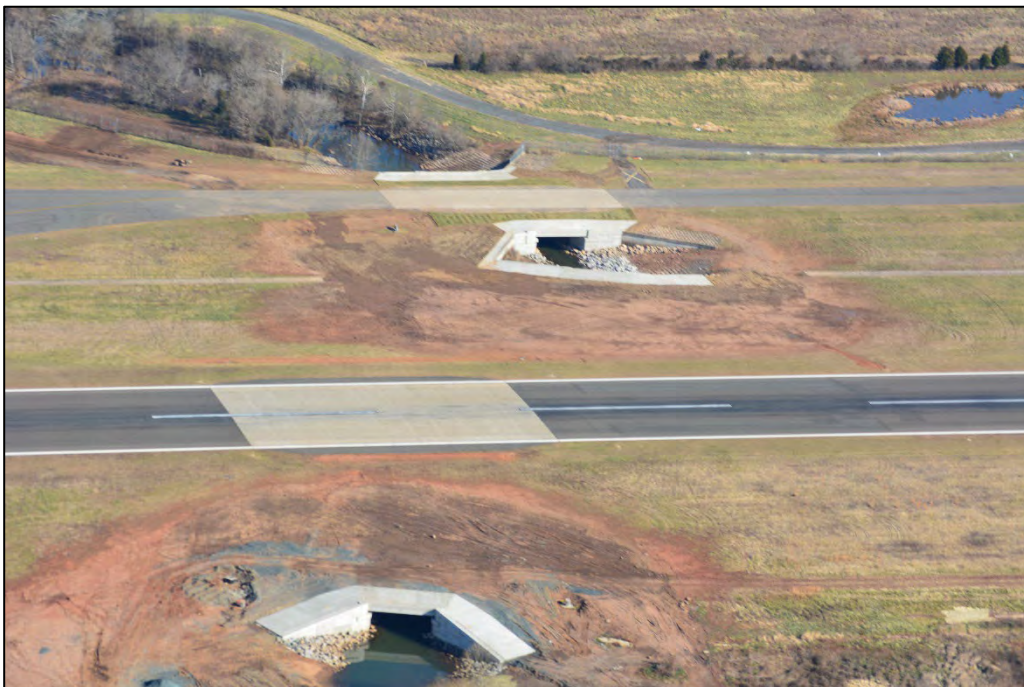
Photograph 16. The new 2014-2015 T/W B and R/W 16L/34R bridge structures (Field Photograph Airport_DSC0191, 2014).
