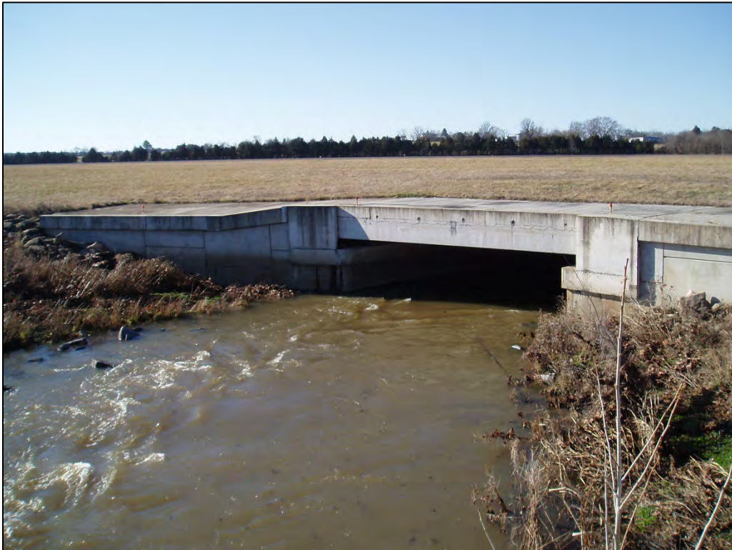
Photograph 18. Looking NE at the bridge structure under R/W 16L/34R (Field Photograph CSW_P0130022, 03/14/2024).
